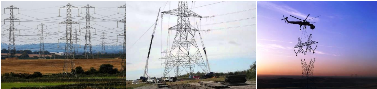
Figure 12. High Power Transmission Lines
